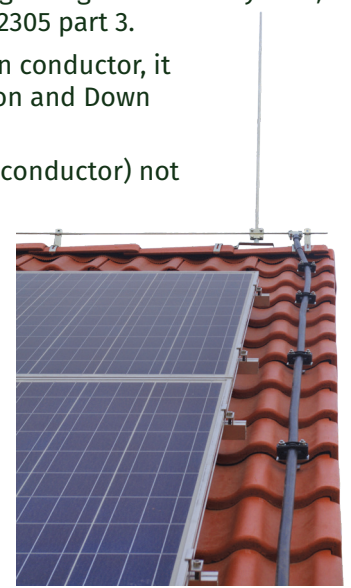
Figure AT:6 - Pitched roof with PV arrays
